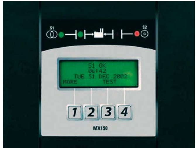
Automatic transfer switch (ATS) control panel inside the front door.
